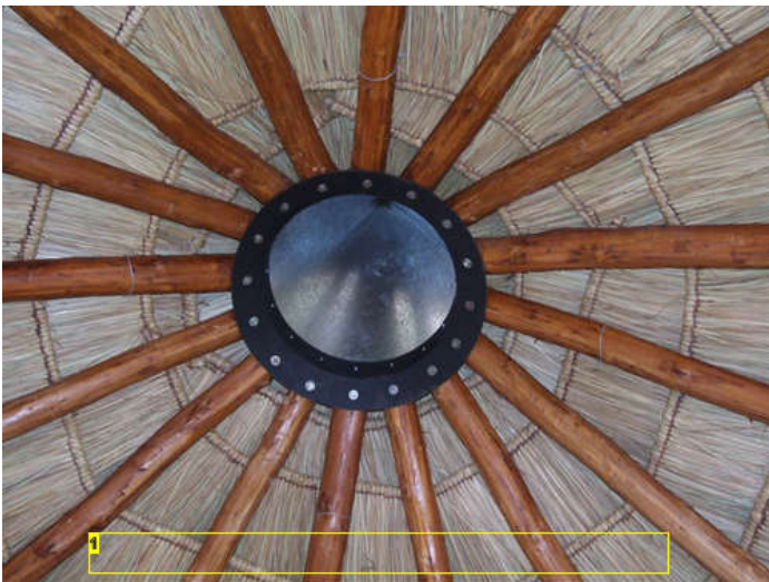
Image Notes 1. Inside View of Roof Showing Compression Ring and Roof Poles
