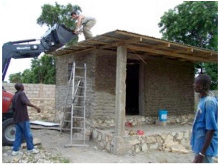
A double 2x4 header attached to the columns supported the porch rafters.
