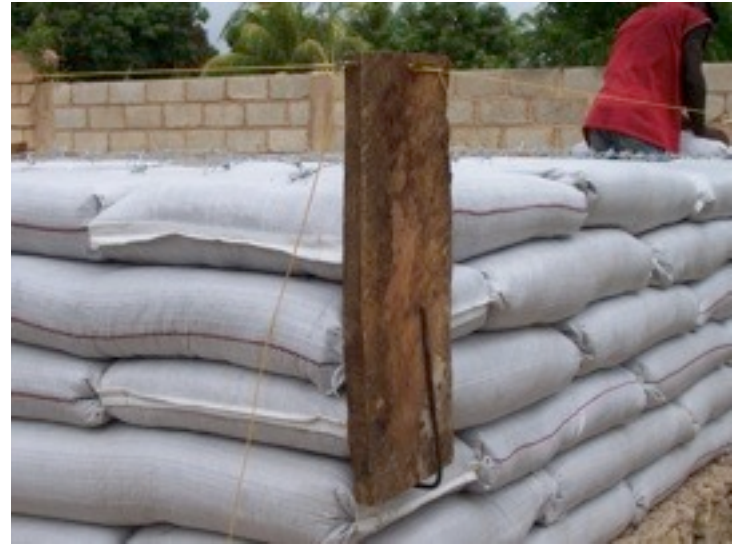
We found a foot long piece of 1/4" bar bent into an "L" helped hold the corner bracket in place.
