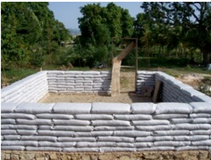
Here is a shot of the house from the back. It was coming up nicely.
