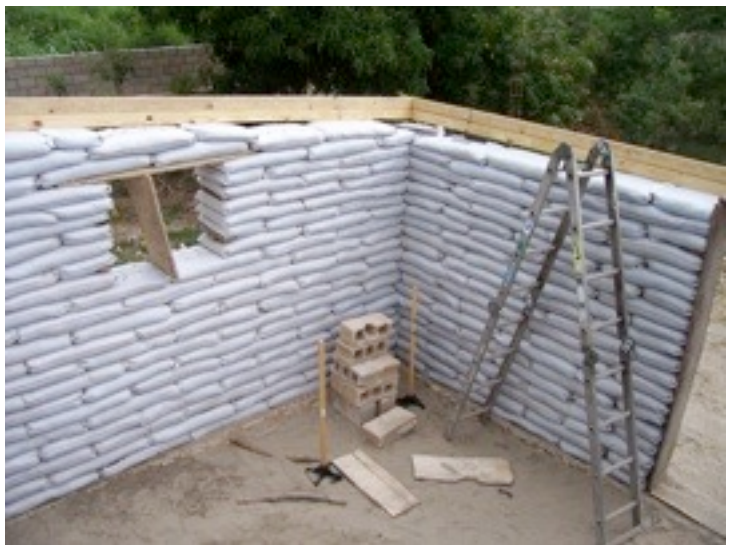
The back wall was 4 coursed higher than the front. Eight 2x4's created the outside of our ring beam form. We placed a temporary support in each window for tamping and pouring the ring beam.
