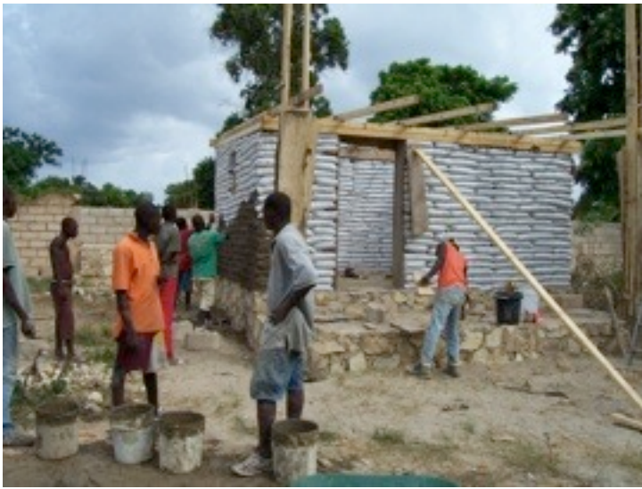
The columns were formed and poured last so we would know exactly how high to make them.
