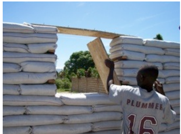
The side forms were removed. The windows and doors will be attached later to the wood cleats placed along the sides of the openings.
