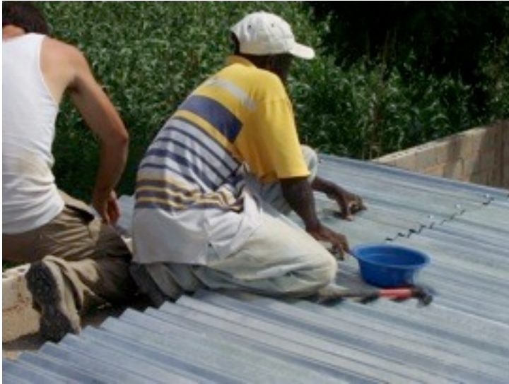
The roofing was nailed down. I had thought of stretching metal banding across the sheets to hold them down in the wind, but opted not to.
