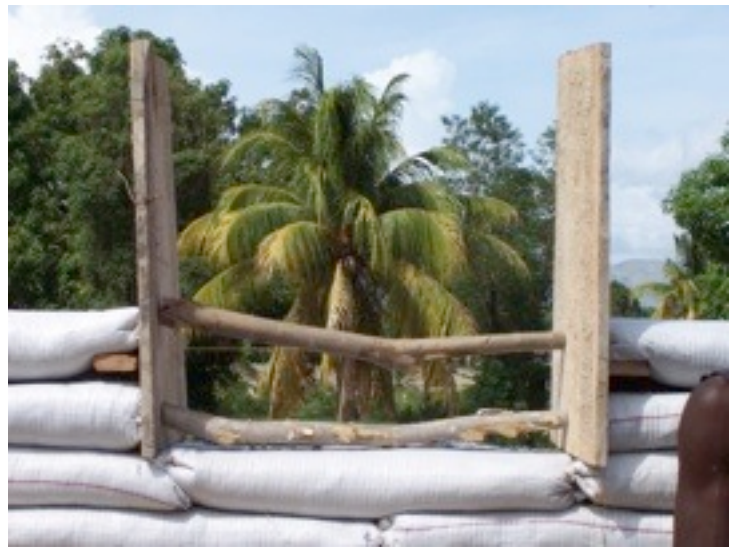
We formed the door and window openings with the wood at hand. They don't need to look pretty, just get the job done.
