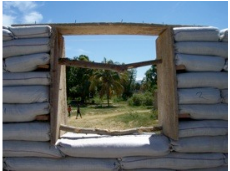
We moved the top spacer up as we went. The wood header protruded past the sides of the window about a foot on each side. Lots of nails in the header kept it from moving.
