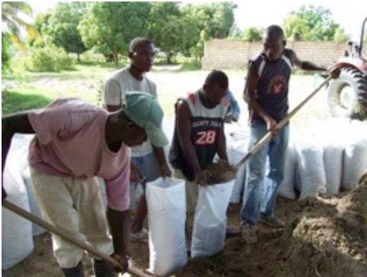
No measuring buckets or funnels kept the project moving quickly. Filling to a line and then tamping to a string seemed to take care of the problem of uneven bags.
