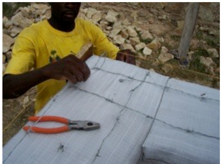
We opted for barbed wire instead of driving rebar through the courses. We used 3 rolls and it was cheaper than the rebar, as well as easier to transport. It also gave the walls tensile strength.
