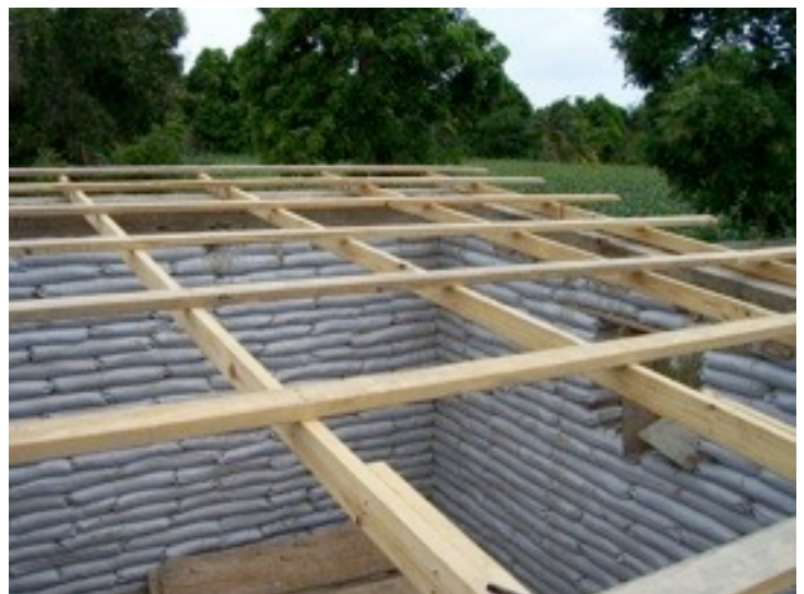
Six rafters seemed adequate and the purlins were placed every 32" to accommodate the 6' long metal sheets.
