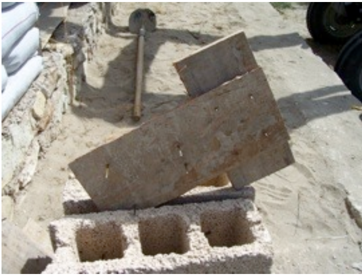
Close up of a wood cleat used along the openings. Lots of nails sticking out the top and bottom insured it wouldn't slip in the wall.
