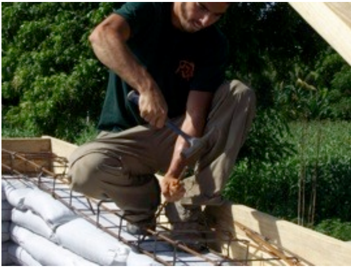
Rebar was placed along the top of the wall and 30" long pieces were driven down at angles and left sticking out 6 inches to connect the concrete beam to the bag wall.
