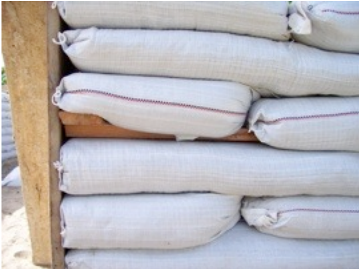
This wood cleat was placed along side the door opening. A piece of plywood with a 2x4 nailed to it would have been nice, but the scrap wood we had worked okay.
