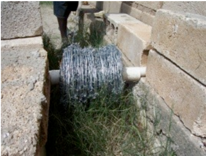
We placed the barbed wire on a make shift dispenser. This allowed two guys to simply pull off a piece and cut it to length.
