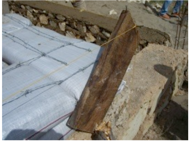
We used blocks of wood with 5 16d nails driven through them at each corner to hold the string for each course. We used a plumb line to set the corner each time. We had to place them at a slant for the first few courses.
