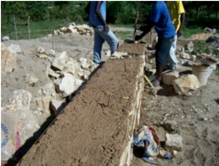
We placed small pieces of rebar every 4 feet or so to keep the first layer of bags from sliding.
