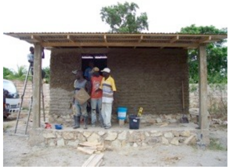
The first coat of plaster was left rough. The second coat will come later and be smoothed to a nice finish.
