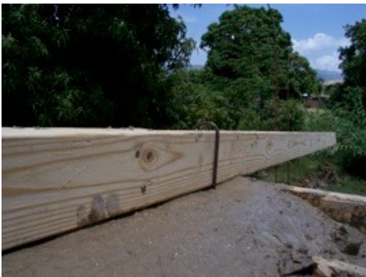
The rafters were set in place as we poured the beam. We did the two side rafters first and then set the others to a string stretched between them.
