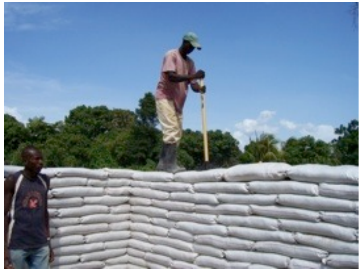
After each course was laid it was then tamped to the string. We found an 8" square tamper worked well. Much bigger and you have to hold it out from your body to keep from hitting your toes. That gets tiring by the end of the day.
