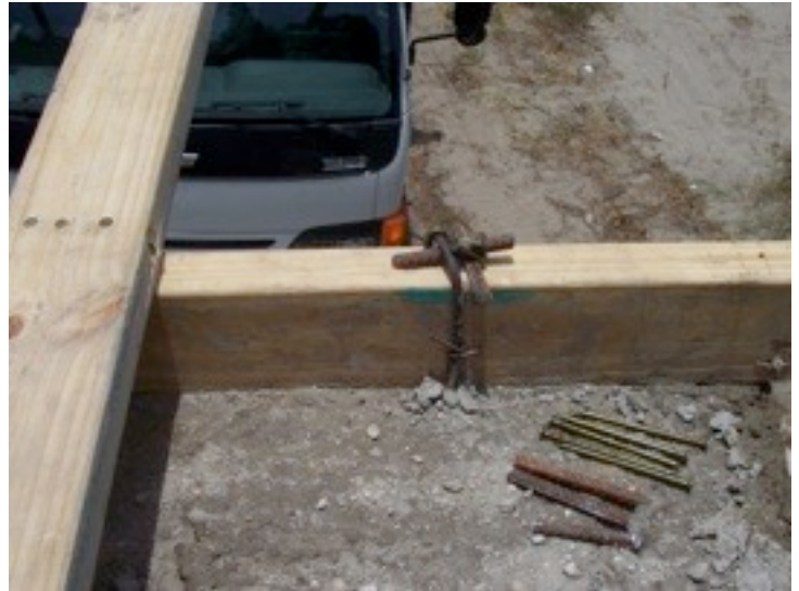
Once the concrete set we tightened the rafters down by driving pieces of rebar between the strap and rafter. We locked it all in place with bent nails.
